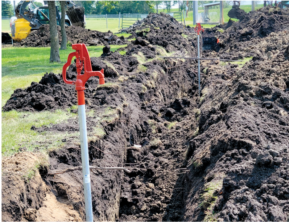
Campground addition coming along City workers and contractors have been busy digging in water lines for the City Park camping addition. (Submitted photo)
