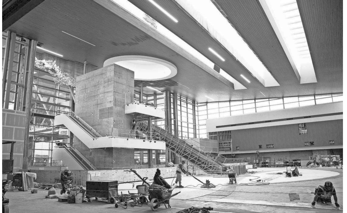
Construction workers build the new main terminal at the Nashville International Airport on Dec. 9 in Nashville. GEORGE WALKER IV / THE TENNESSEAN
