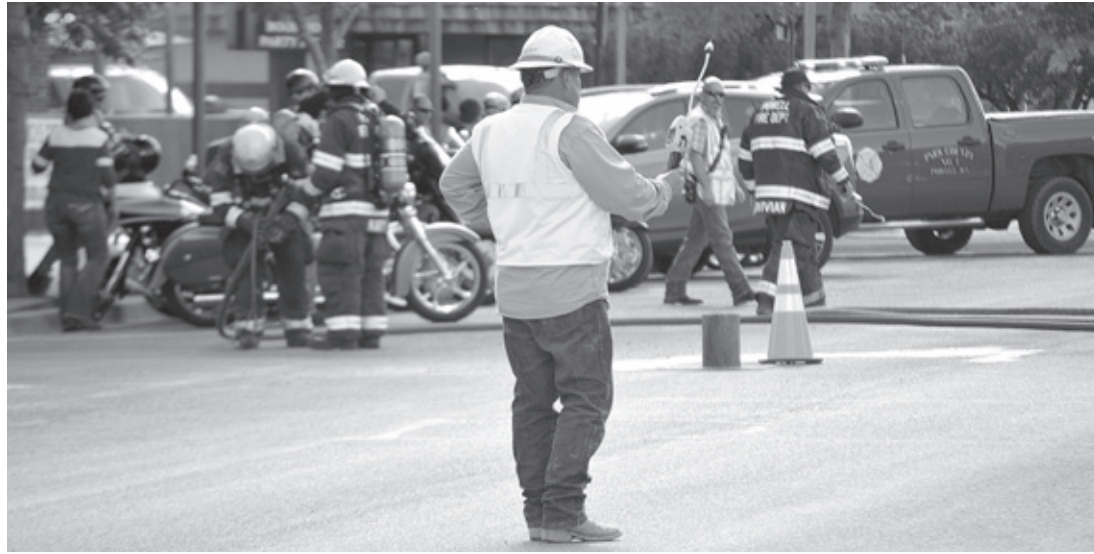
An MDU worker monitors the air quality downwind of the spot (marked by a cone) where a contractor accidentally bored into a 6-inch natural gas line on First Street Thursday afternoon. Because a specialized piece of equipment was required, it took nearly nine hours for crews to shut off the leaking line. Tribune photo by CJ Baker
