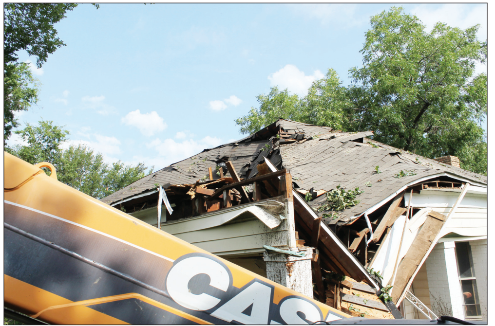
The tree removal crew worked quickly and with the branches removed, the severe damage to the roof on this Johnson Street house could be seen.
